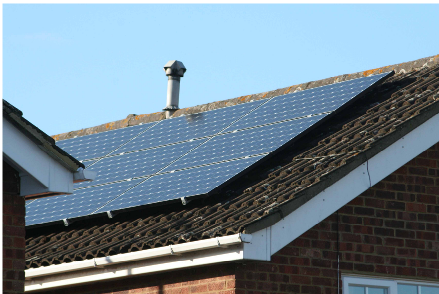
A 2.5kW peak Solar PV system
